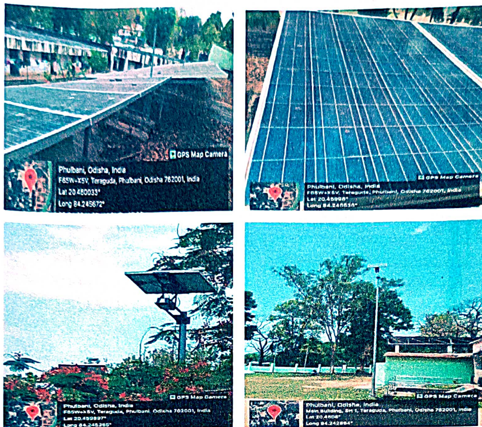
Figure 4. Solar installations of the college campus.
